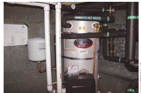
The Erkelens' smallest array, with four Schüco collectors and a single Phoenix storage tank, supplies nine apartments in an older building.
